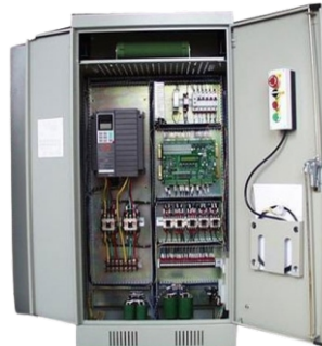
Integrated Lift Controller
